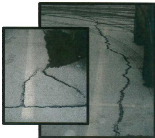
Damaged parking areas
